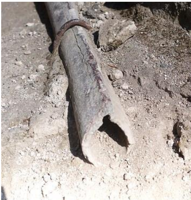
Figure 37 An example of lead pipe strapping from Pompeii (image downloaded from flickr)
